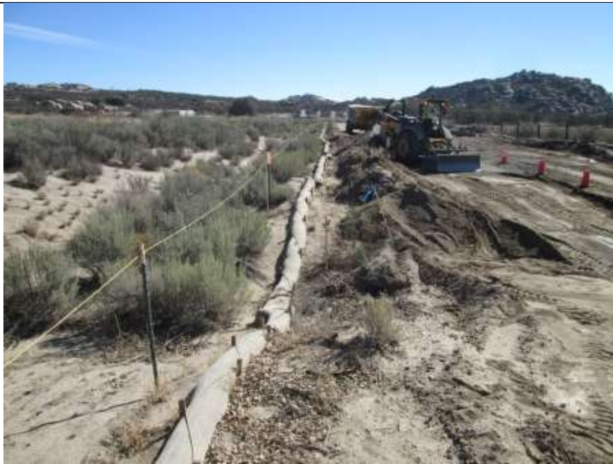
Photo 2: Along Section 1 of the underground transmission line, excavation in preparation for the storm drain pipe installation was observed being conducted within delineated work limits. Erosion control devices were observed intact in accordance with MM-HYD-1 and water was
