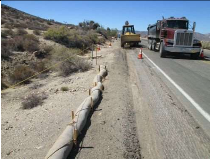
Photo 1: During road improvements along Section 3 of the underground transmission line, crews were observed staying within the work limits and erosion control devices were observed intact in accordance with MM-HYD-1.
